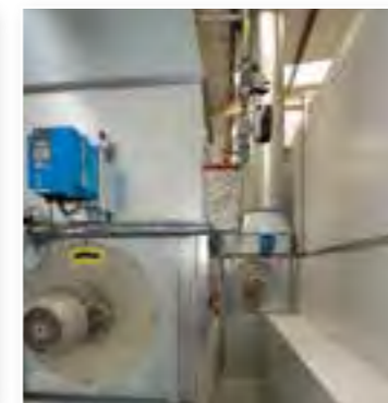
ENERGY-EFFICIENT AIR HANDLING PLANT
