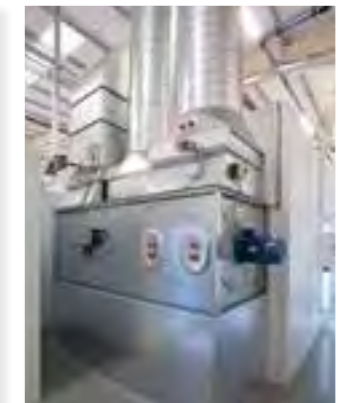
ENERGY-EFFICIENT AIR HANDLING PLANT
