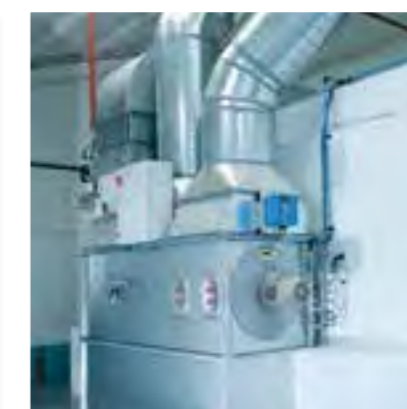
ENERGY-EFFICIENT AIR HANDLING PLANT
