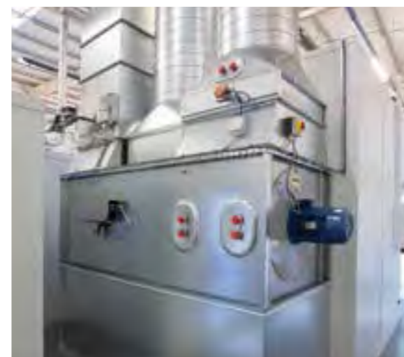
ENERGY-EFFICIENT AIR HANDLING PLANT
